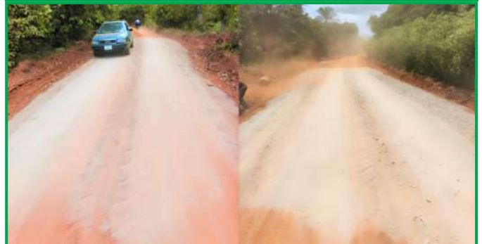
21KM ROAD GRADED FROM OKOMU MAIN GATE TO GBELEBU, AND MADAGBAYO COMMUNITIES
