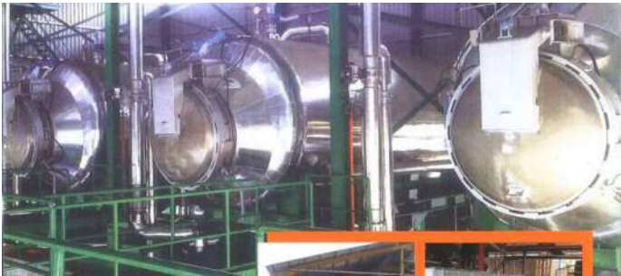
FIRST EVER TILTING STERILIZER IN AFRICA INSTALLED IN OUR MAIN ESTATE OIL MILL
