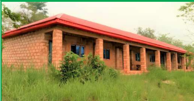
FIRST PHASE OF THE CONSTRUCTION OF A BLOCK OF CLASSROOMS AT ORHUA COMMUNITY
