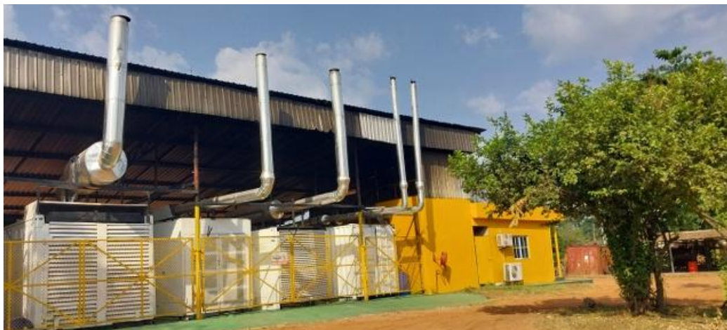
Plate 2.7: Generating sets at the Main Estate Powerhouse
