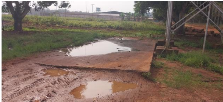
Plate 4.4b: Caved in Inspection Chamber
