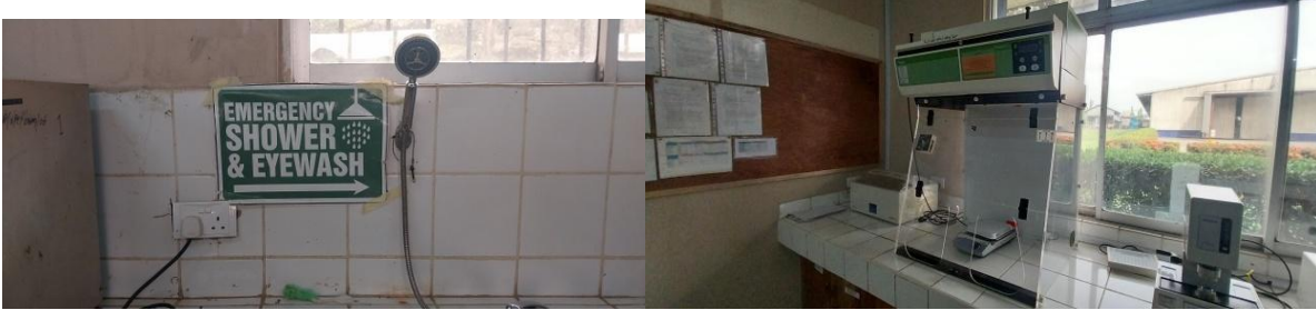
Plate 4.2: Emergency Shower/Eye Wash and Fume Cupboard
