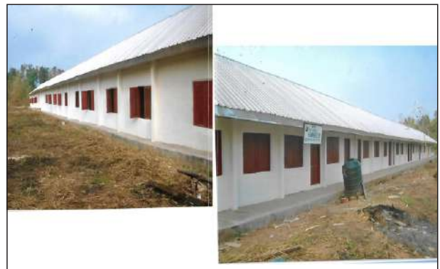
FIRST PHASE OF THE CONSTRUCTION OF IDIA SECONDARY SCHOOL, OKE COMMUNITY, UHUNMWONDE LGA
